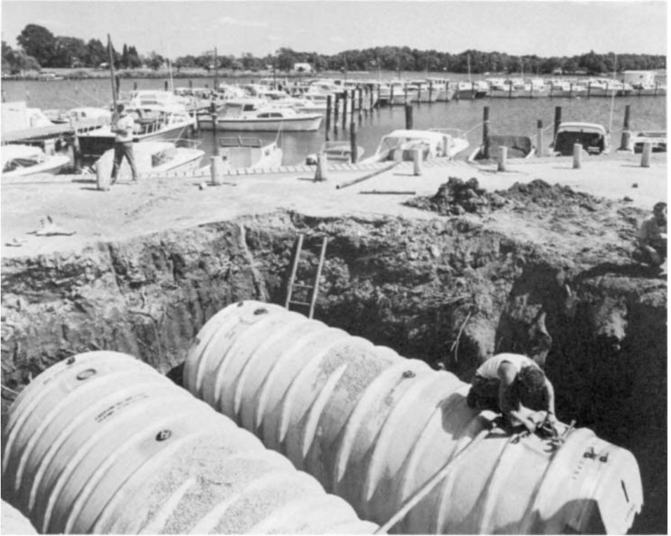
Figure 12.12 Glass fiber–polyester 4000 gallon (15.2 m 3 ) tanks in a highly corrosive environment (salt water).
